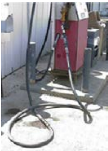
X Evidence of leak shown at hose connection
