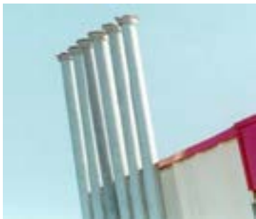
Example of vent pipes secured to a wall
