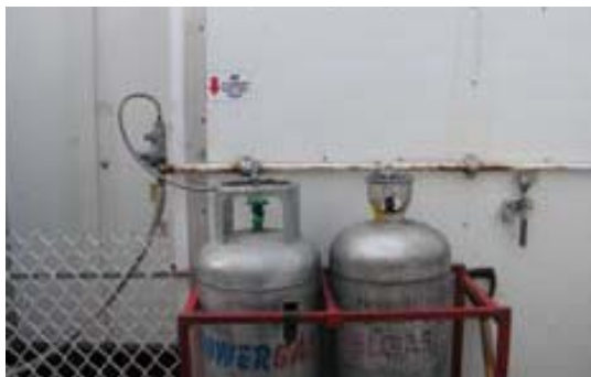
Secured and clear of combustibles
